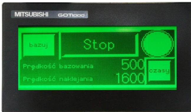
Photo no 10. Main panel II
