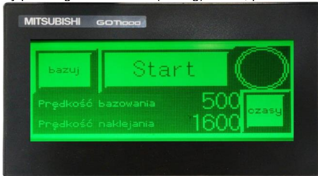
Photo no 8. Main controlling panel
