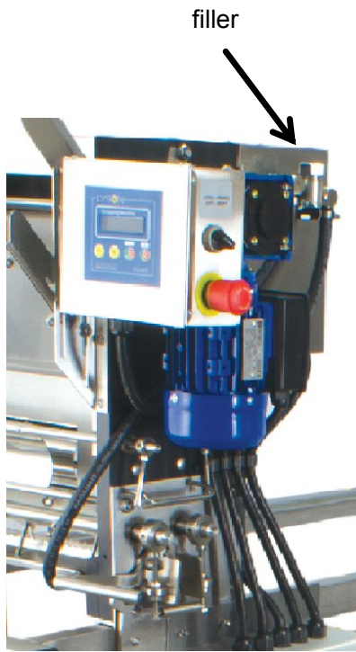
Fig.18. The place where the filler is located to refill the tank with fluid.
