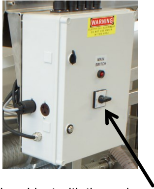
Fig 22. Power supply cabinet with the main switch
