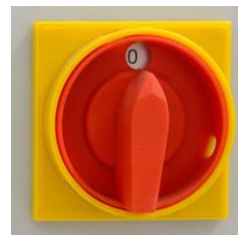
Fig 29. Switch in "0" position
