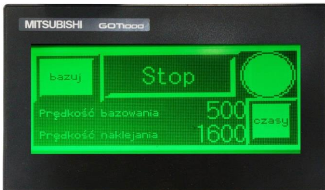
Photo no 14. Main panel II
